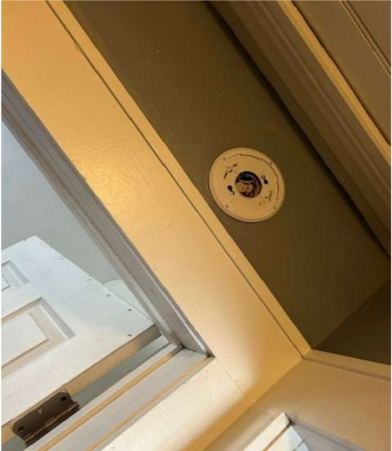
10 shows the missing smoke alarm
