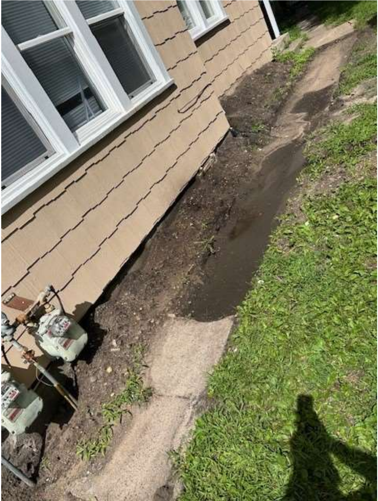
- 4-5 show a large vacant space where a sidewalk once was and the erosion that is happening in its absence, a slipping, tripping, and falling hazards.
